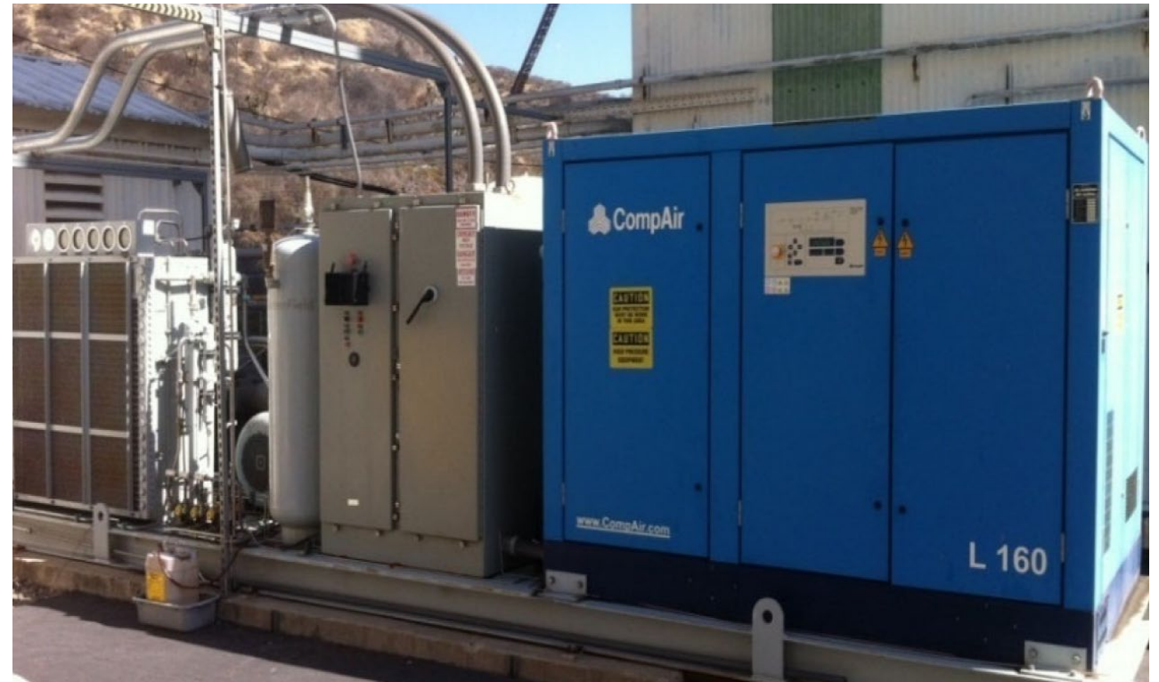
Two stage air compressor skids (General Atomics 2021)
