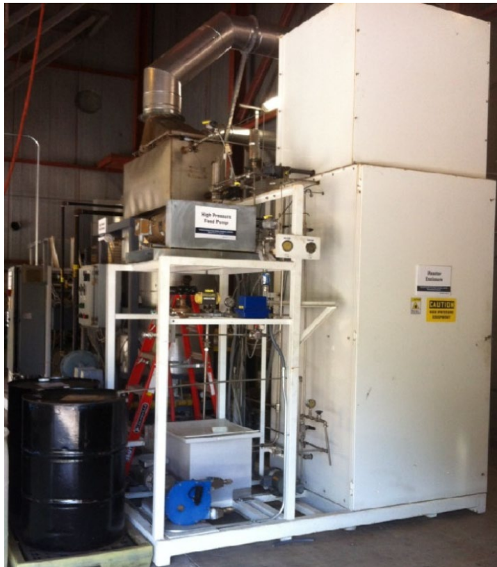
SCWO skid used for validation testing (General Atomics 2021)
